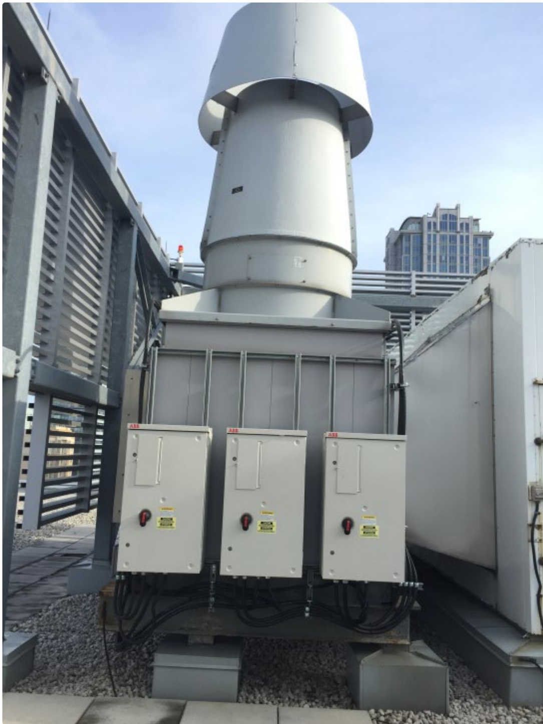
Exhaust Fan with New VFDs Installed
