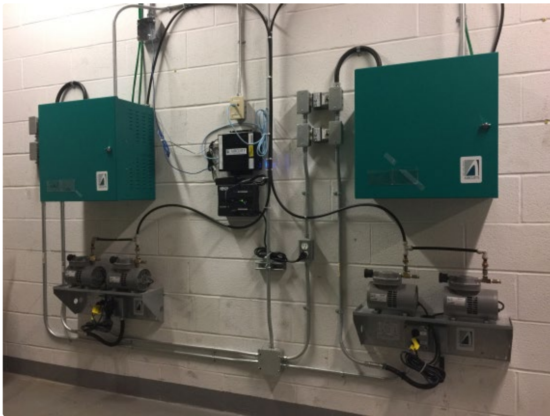
Aircuity Sensor Suites Installed by Airgenuity
